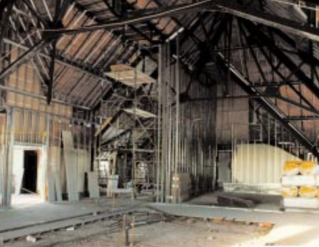
The mezzanine level in Lyons Hall is accented with raised ceilings and exposed trusses.
