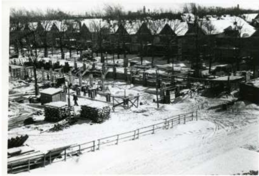
This photo shows the early construction stage for the Horan-O'Donnell Science Building. The houses along Hughes Ave in the background give a familiar appearance to the scene.
